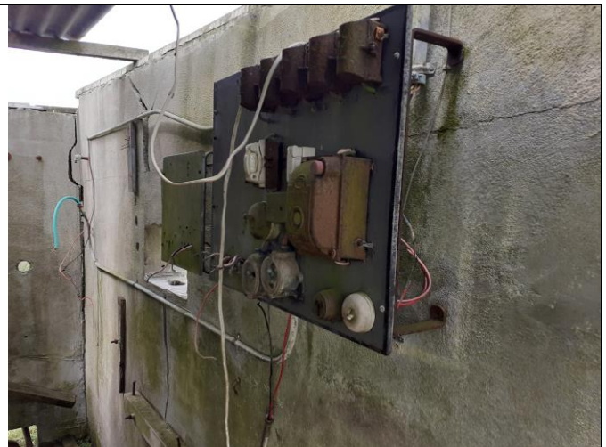
Both the concrete shed and the dilapidated corrugated iron shed contained a circuit board which has the potential to contain asbestos.
