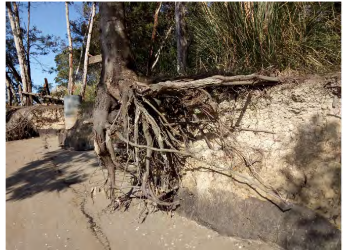
Photo 13: Erosion at the brickworks site. Planting is unlikely to slow erosion as wind-driven waves can undermine the root plate.
