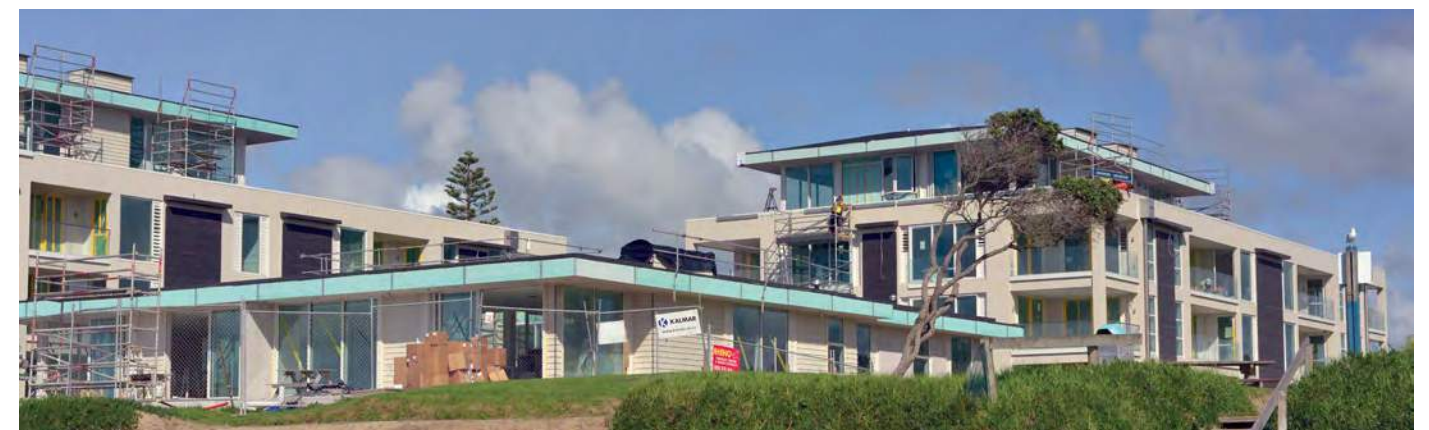
Apartment redevelopment of the Sands Motel site demonstrates the continued market for luxury beachfront apartments.
