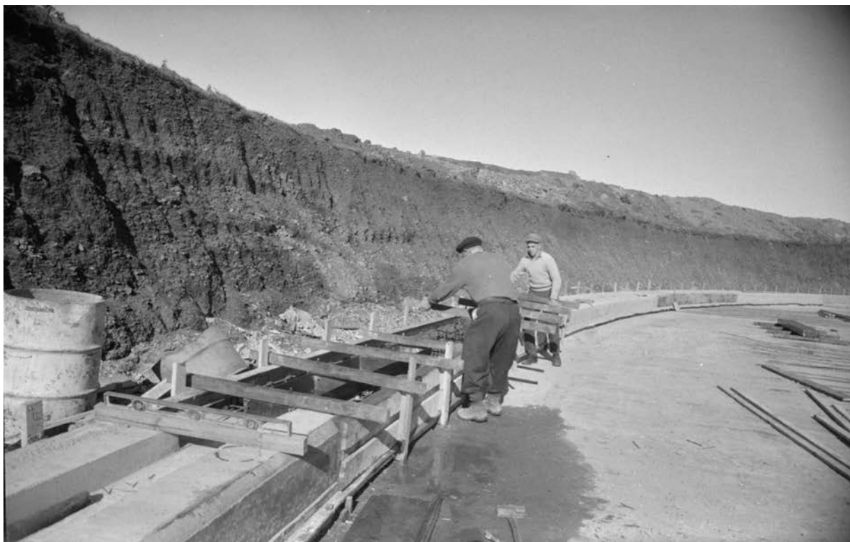
Figure 35: Showing the Mount Roskill Reservoir under construction July 1962, Sir George Grey Special Collections, Auckland Libraries, 580-6549.
