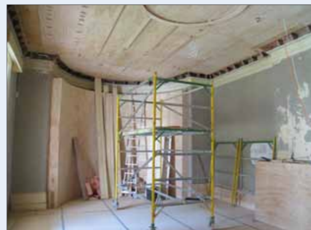
Extensive restoration of ceilings and interior finishes was undertaken in 2009. Image courtesy of Matthews & Matthews Architects Ltd.
