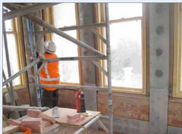
Steel plate frame being installed to strengthen the tower, September 2009. Image courtesy of Matthews & Matthews Architects Ltd.
