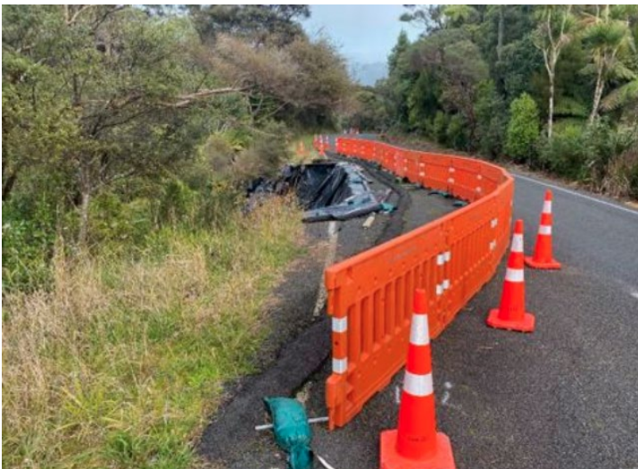
Slip from August 2022 storm
