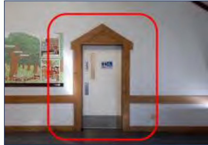
Left: Internal bathroom door to be rehung to open outwards
