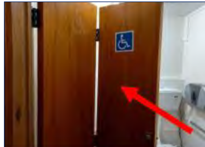
Left: Accessible bifold toilet door to be replaced with new compliant door.
