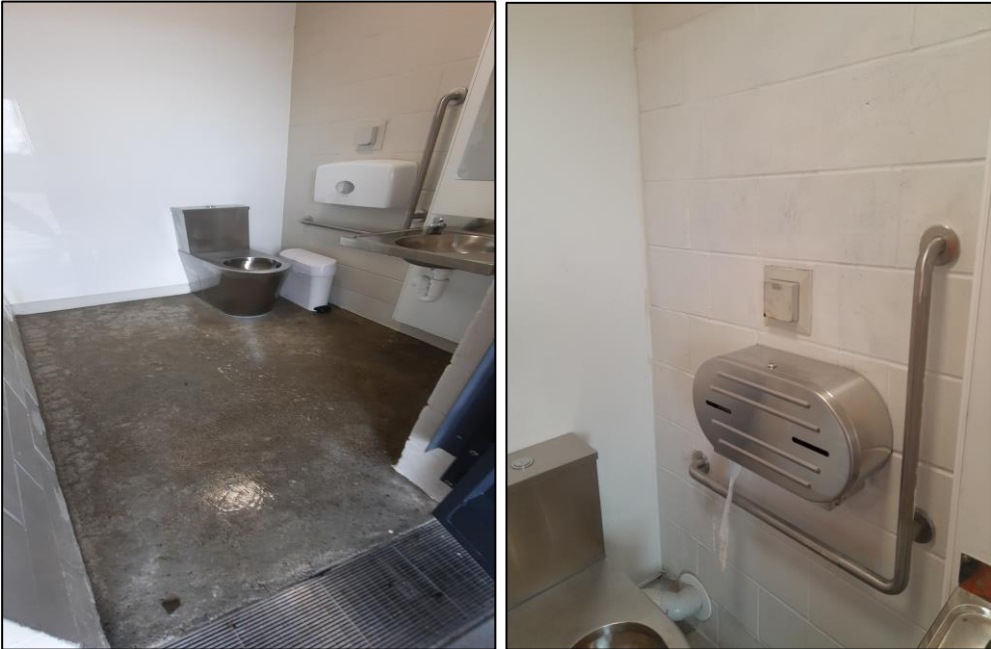
Stainless steel toilet roll holder installed due to continued vandalism
