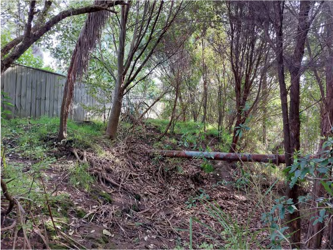
Picture 9 – 150Ø Wastewater pipe
