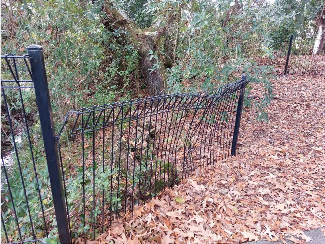
Picture 3 – Damaged steel barrier at Glen Eden Picnic Ground
