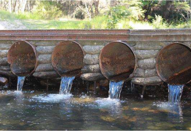
Photo: Instream barriers, such as perched culvert, can prevent inanga migration
