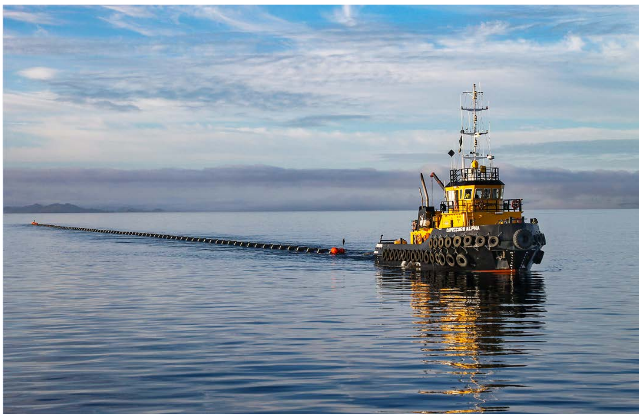
The Army Bay wastewater outfall pipeline project: this photo, taken by Watercare Projects Manager, John McCann, won the Best Photo in Water New Zealand's 2020 Photo Competition.
