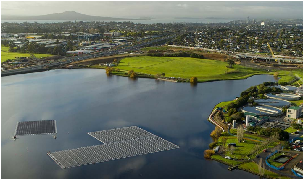
The final piece of the floating solar array at our Rosedale Wastewater Treatment Plant being towed into place
