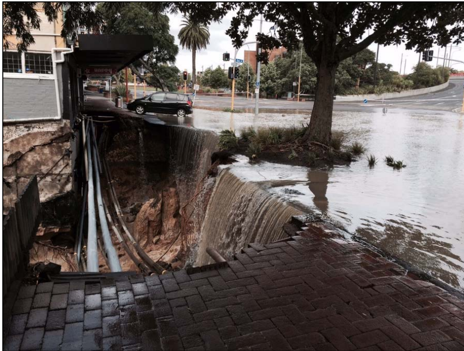
Storm flooding resulted in Watercare water assets being damaged Great North Road, New Lynn
