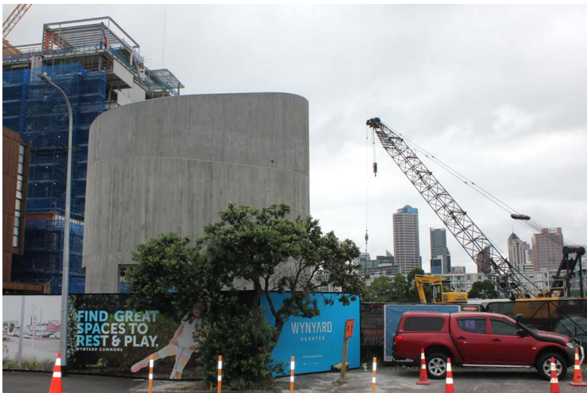
Watercare's new pump station and rising main at Wynyard Quarter is nearing completion
