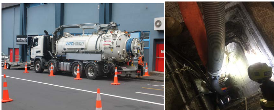
Watercare helped the Newmarket Olympic Pool clear a private blockage, 15 metres under the building
