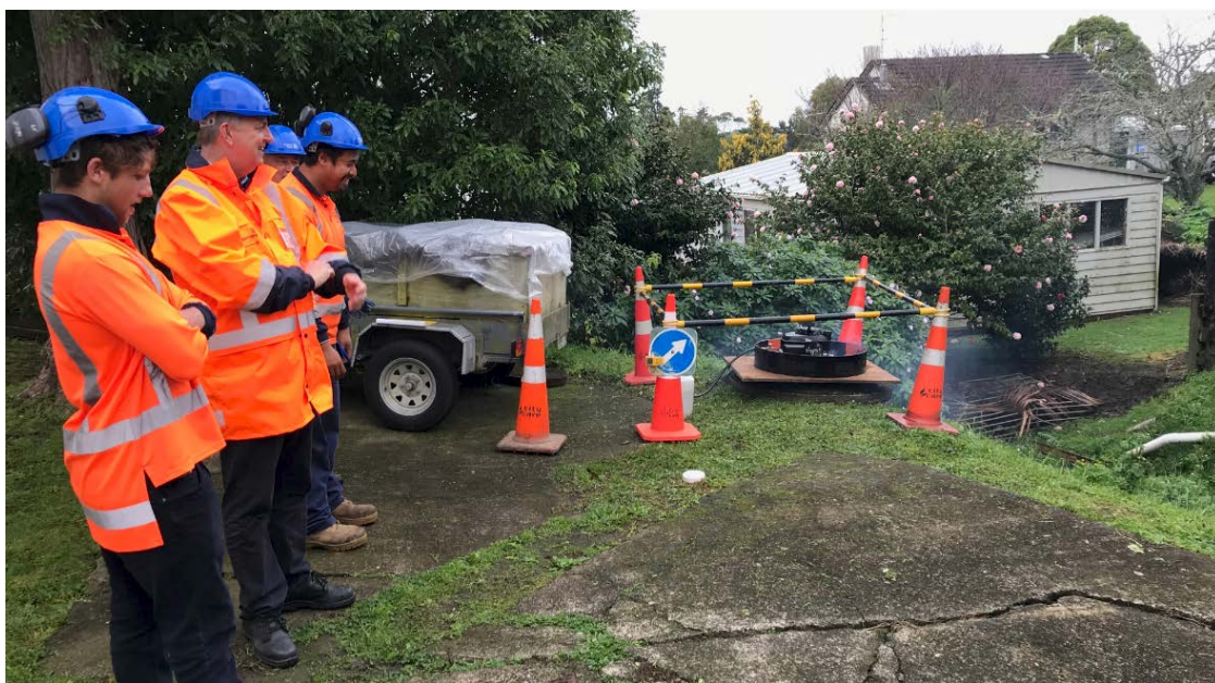
Watercare team conduct Inflow and Infiltration testing in Glen Innes to locate non-compliant connections
