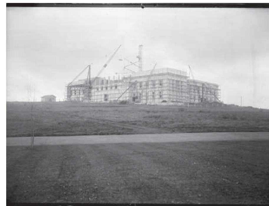
20 May 1927 - Showing the north and west faces of the Auckland War Memorial Museum under construction. Sir George Grey Special Collections, Auckland Libraries, 1-W862.
