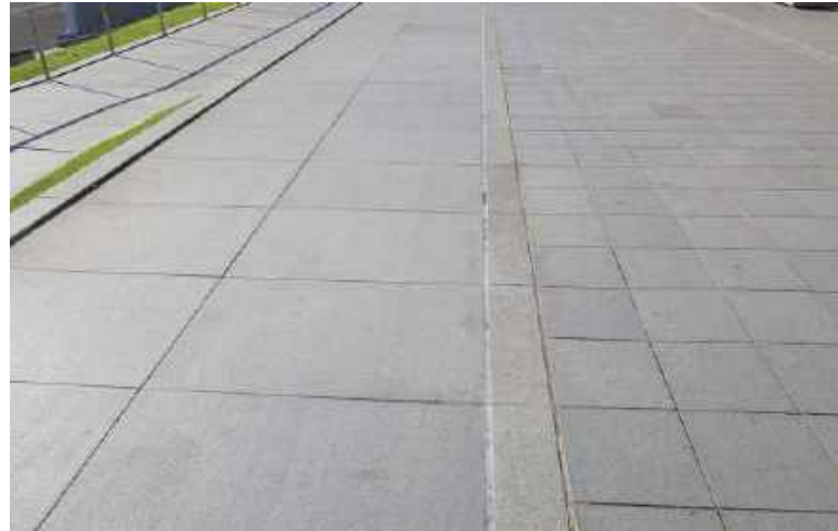
Bluestone paving - for use in new civic spaces surrounding the Museum Notes: materials and details to match existing paving north of Museum
