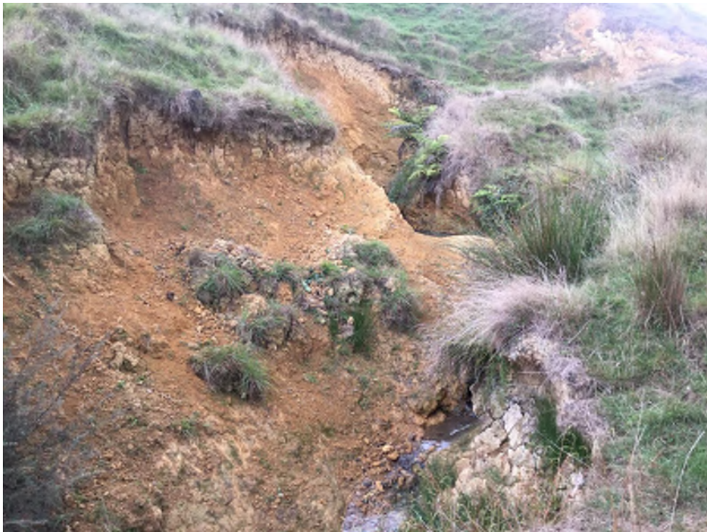
Figure 10: Erosion hotspot alongside a stream channel edge.
