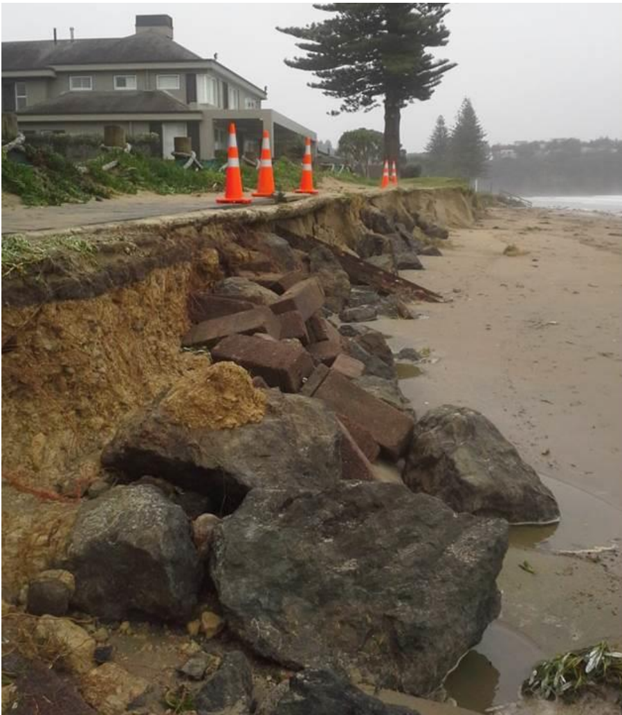
Figure 2: Orewa Beach storm damage 2014 1
