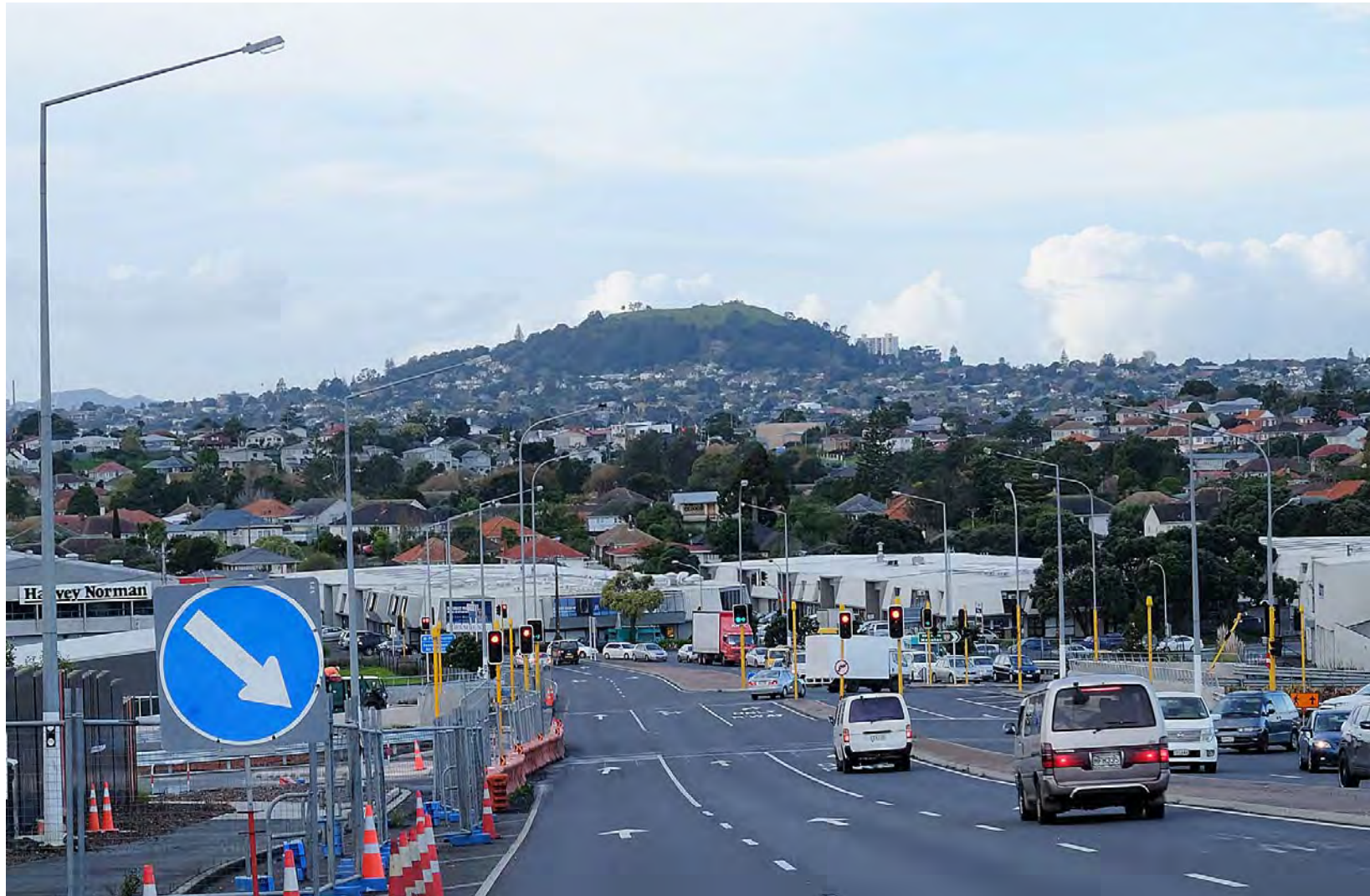
View R01: Photo 3 of 4 Looking From The Maoro Rd Overbridge Towards Mt Eden (75mm lens equivalent) (This photograph is indicative only; field based analysis is required for assessment purposes)
