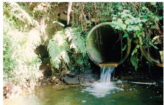
FIGURE 8 Example of a perched culvert, a common barrier to fish passage. Native fish are unable to leap the vertical distance required to enter the culvert and continue migrating upstream. (Source: ARC).
