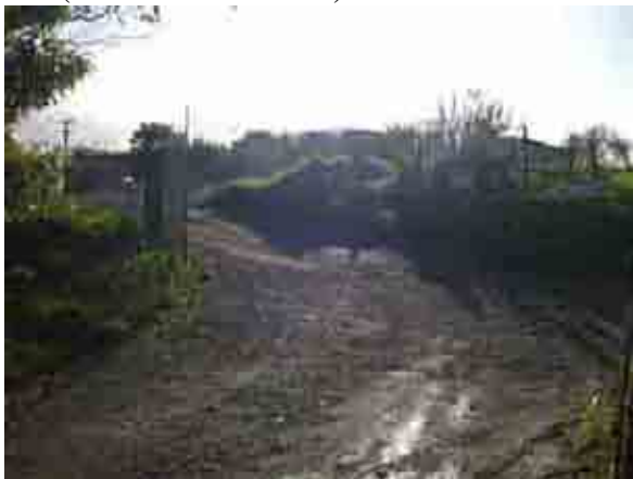
Photo 6. Adams Drive entrance to contractor depot at 1251 Paerata Road. Depot contains stockpiles of assorted material and filling has occurred.
